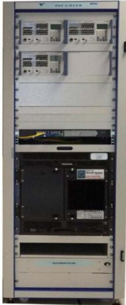
Figure 5: Example of a VHF data link rack
